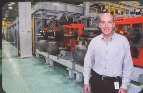
This $50 million machine produces United Solar Ovonic solar laminates. Incorporating a huge array of equipment, it's over 50 meters in length.
